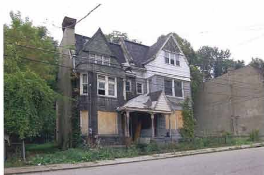
and buildings in deteriorated condition.
