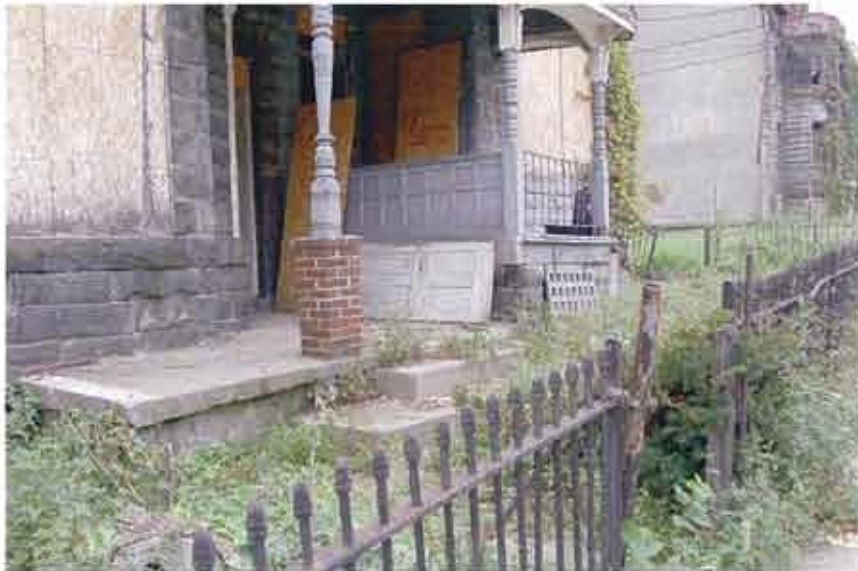
deteriorated sidewalks, front yards, porches...
