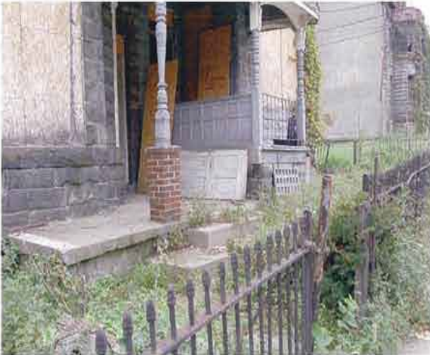
deteriorated sidewalks, front yards, porches...
