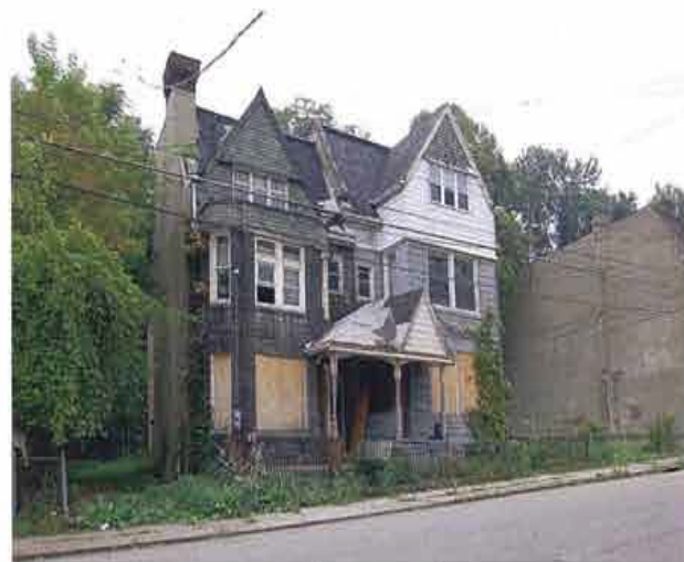
and buildings in deteriorated condition.
